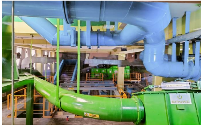
Automated Waste Management Facility
